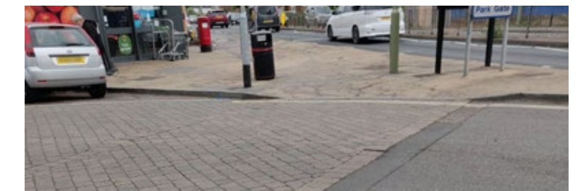
Z2.4.1 Poor crossing on Middle Road junction with A27
